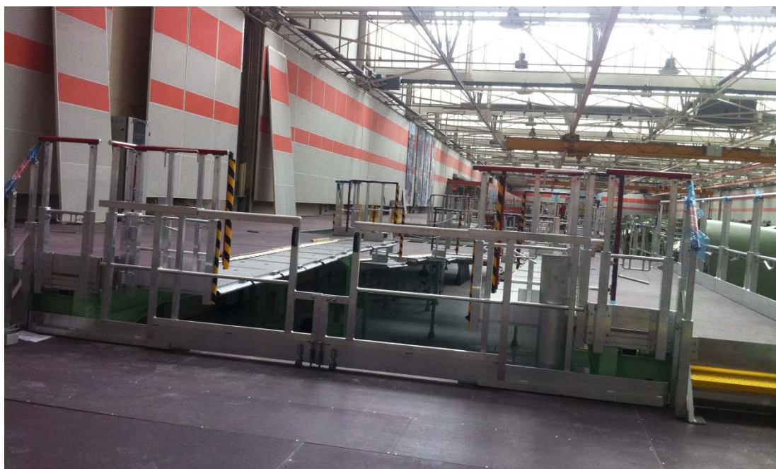
Platform – rear side view. Woods panels – brown, anti-sliping – white color painting for more lightness under the platform.
